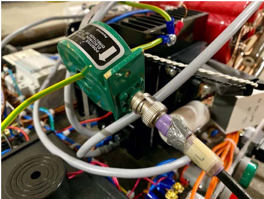
Figure 16: A current transformer was used to measure the secondary currents \hat{I}_2 and the resonant frequency f at ground.
