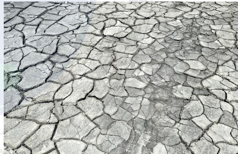
滾水坪泥裂圖2
